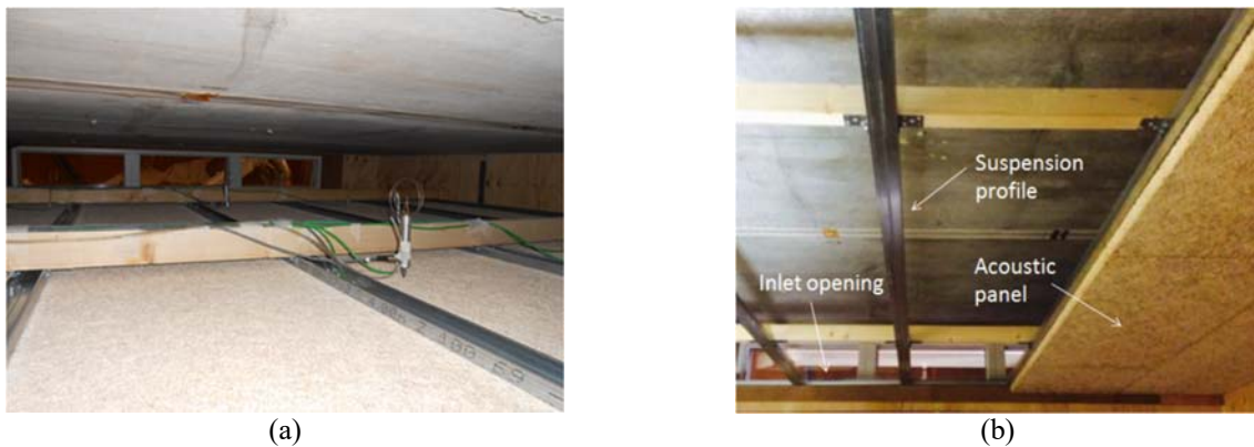
Figure 11: Overhead plenum and diffuse ceiling setup [2]
